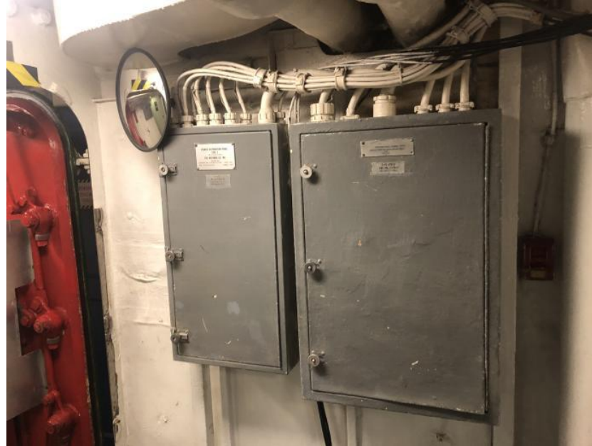
Power Panel (Photo by Norbert Doerry)
