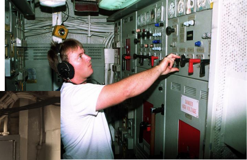
Switchboard (Image is in the public domain)
