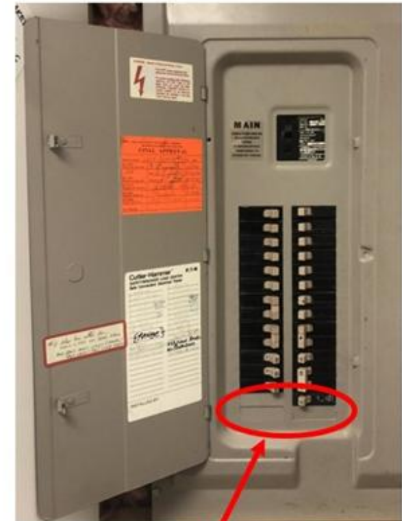
Spare Circuit Breaker Slots
